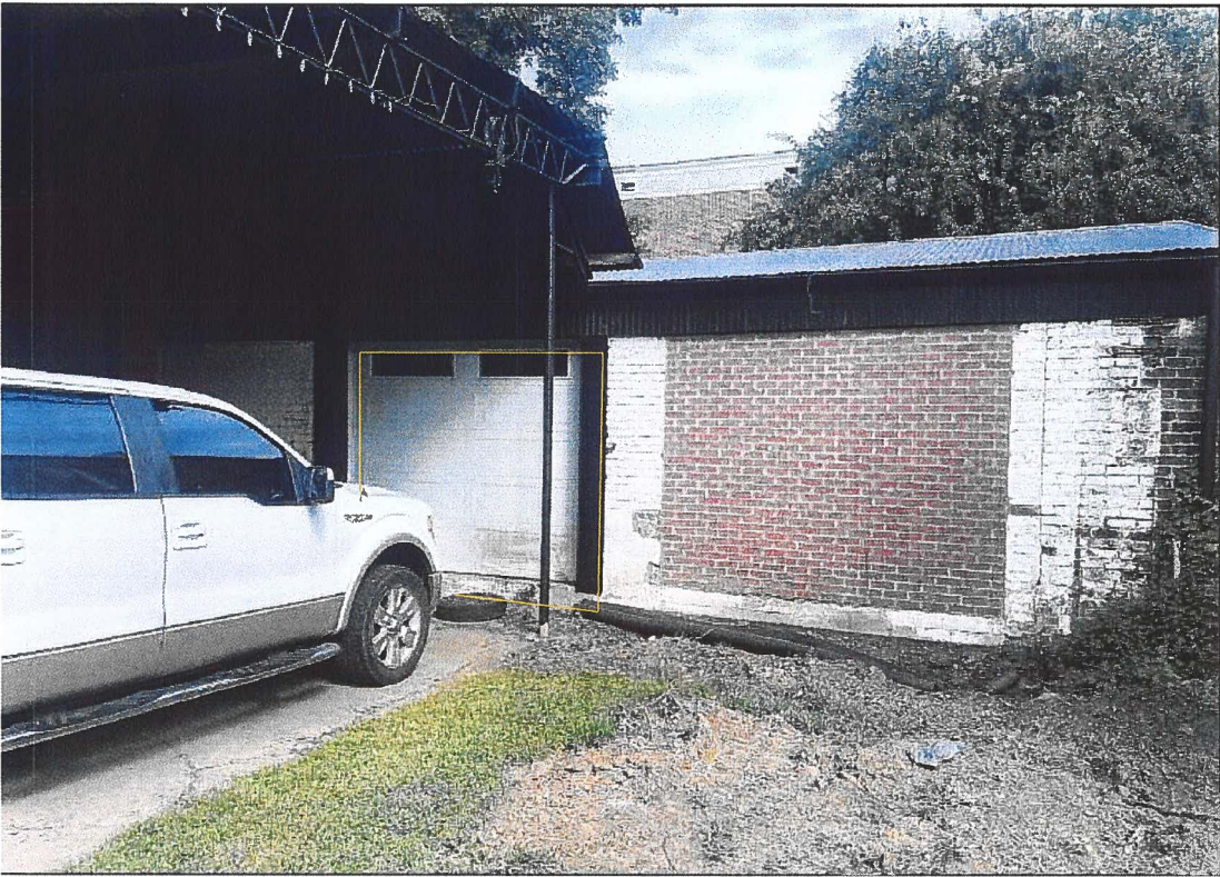
Replace door to match glass and metal overhead door to the left.
