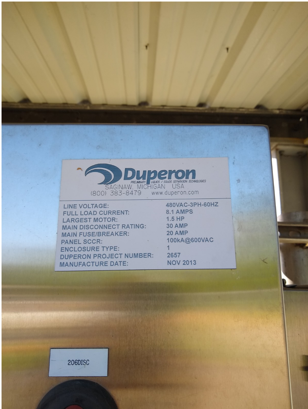
Figure 4. Existing control panel.
