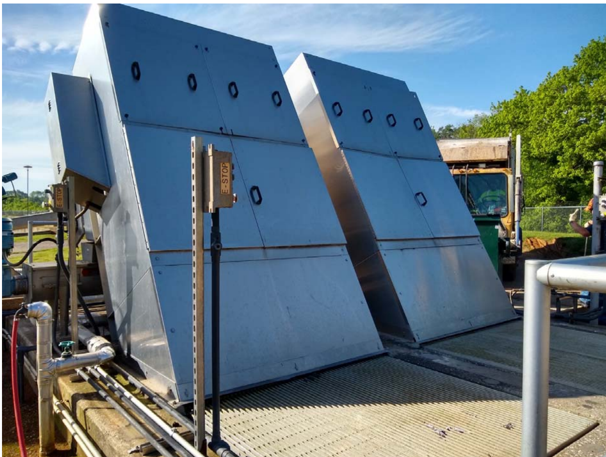
Figure 2. Existing bar screen
