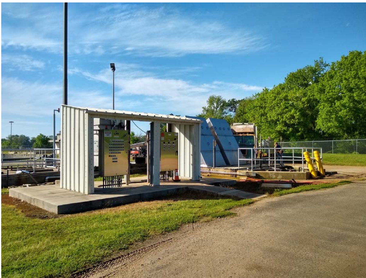
Figure 1. Existing bar screen and control site
