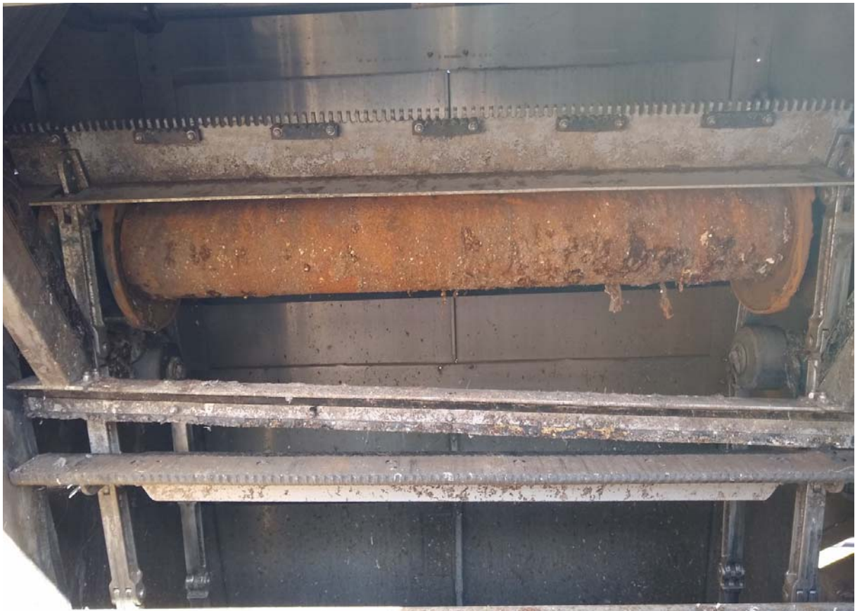
Figure 5. Existing bar screen rake and mechanisms (to be replaced).
