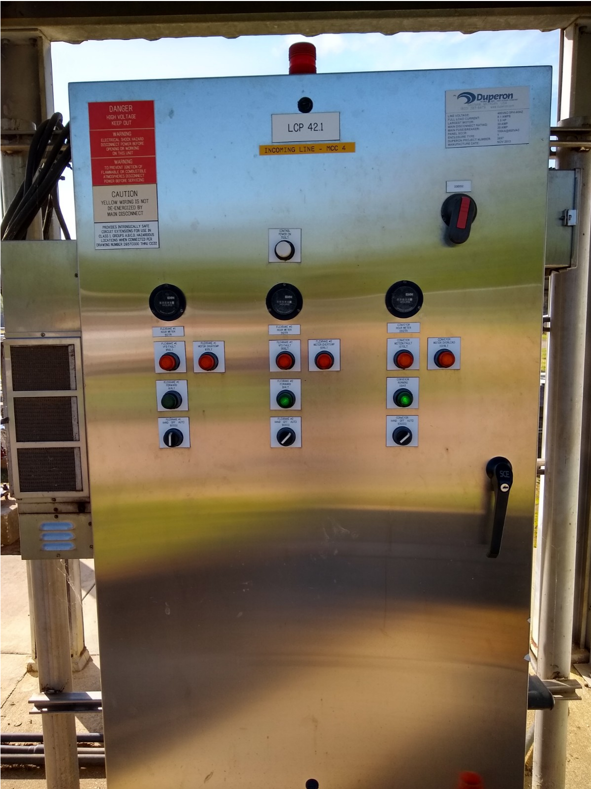
Figure 3. Existing control panel
