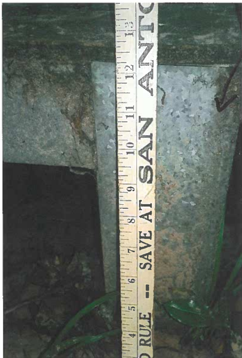
12 INCHES OF TABLE'S FRONT LEG IS BURIED IN SAND
