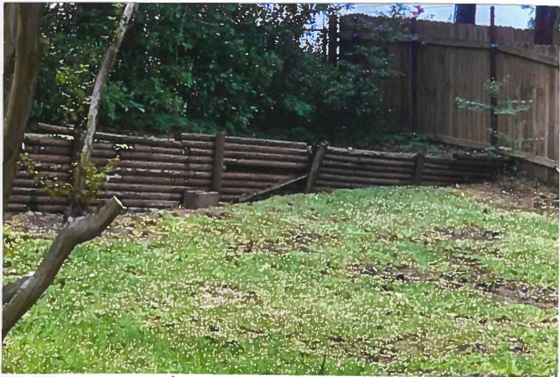
RETAINING WALL IS COMING DOWN DUE TO RUN OFF HAVE A $13,500.00 BID TO REPLACE
