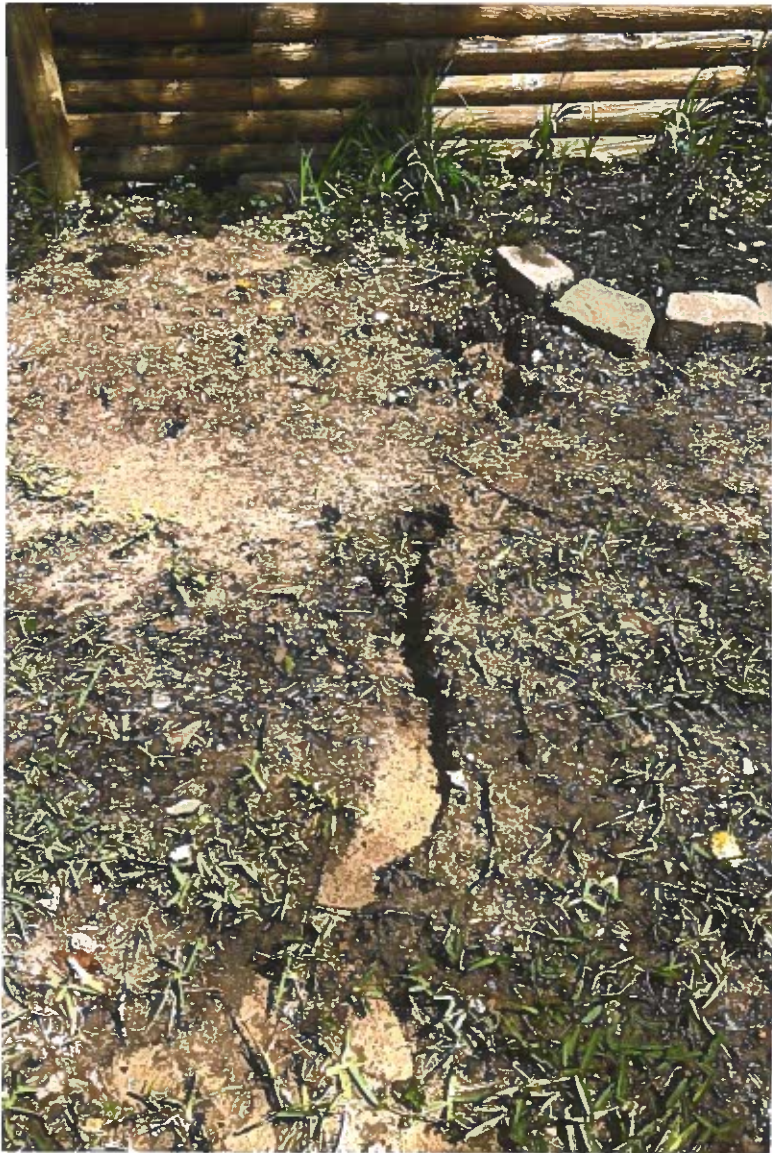
Water comes over and under retaining wall
