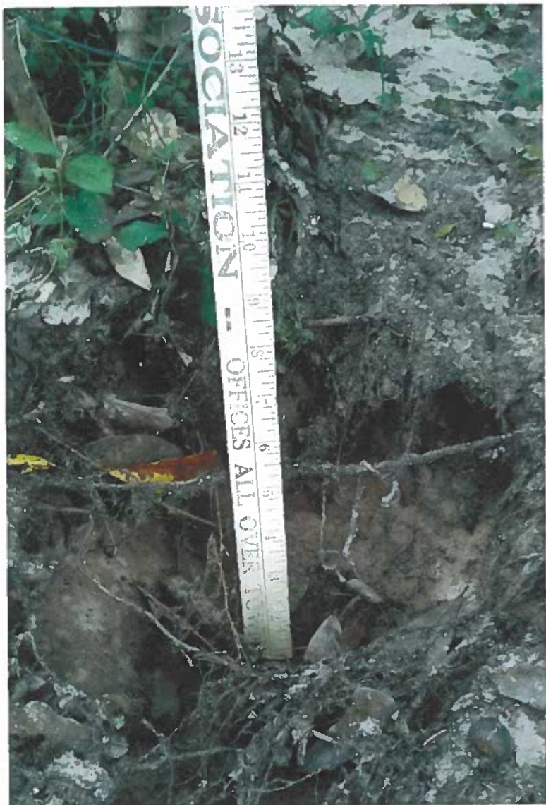
13" WASHOUT - ONE OF MANY
