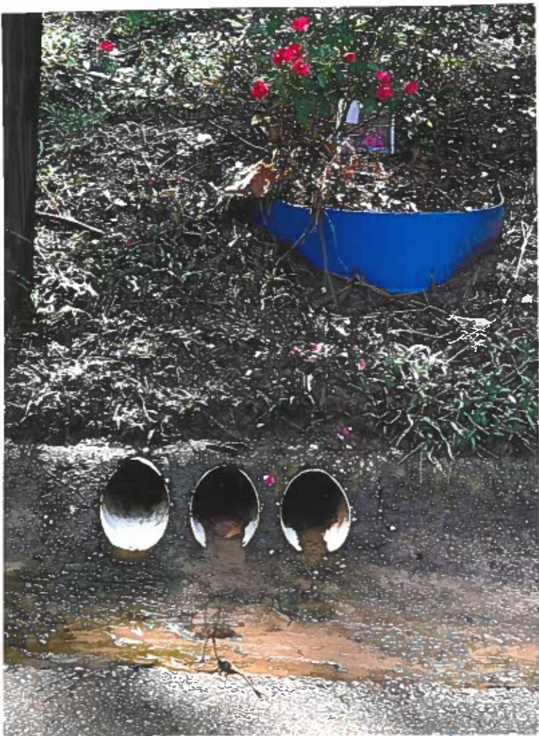
3 CATCH BASINS FILLED WITH SAND - HAVE TO REPLACE
