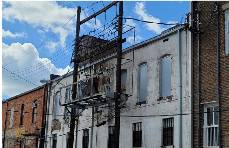
Above ground alley utility in Downtown
