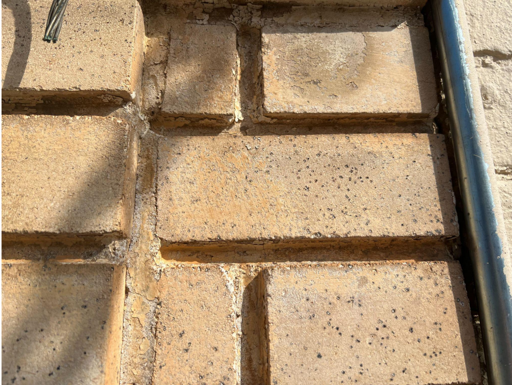
Paint in grout
