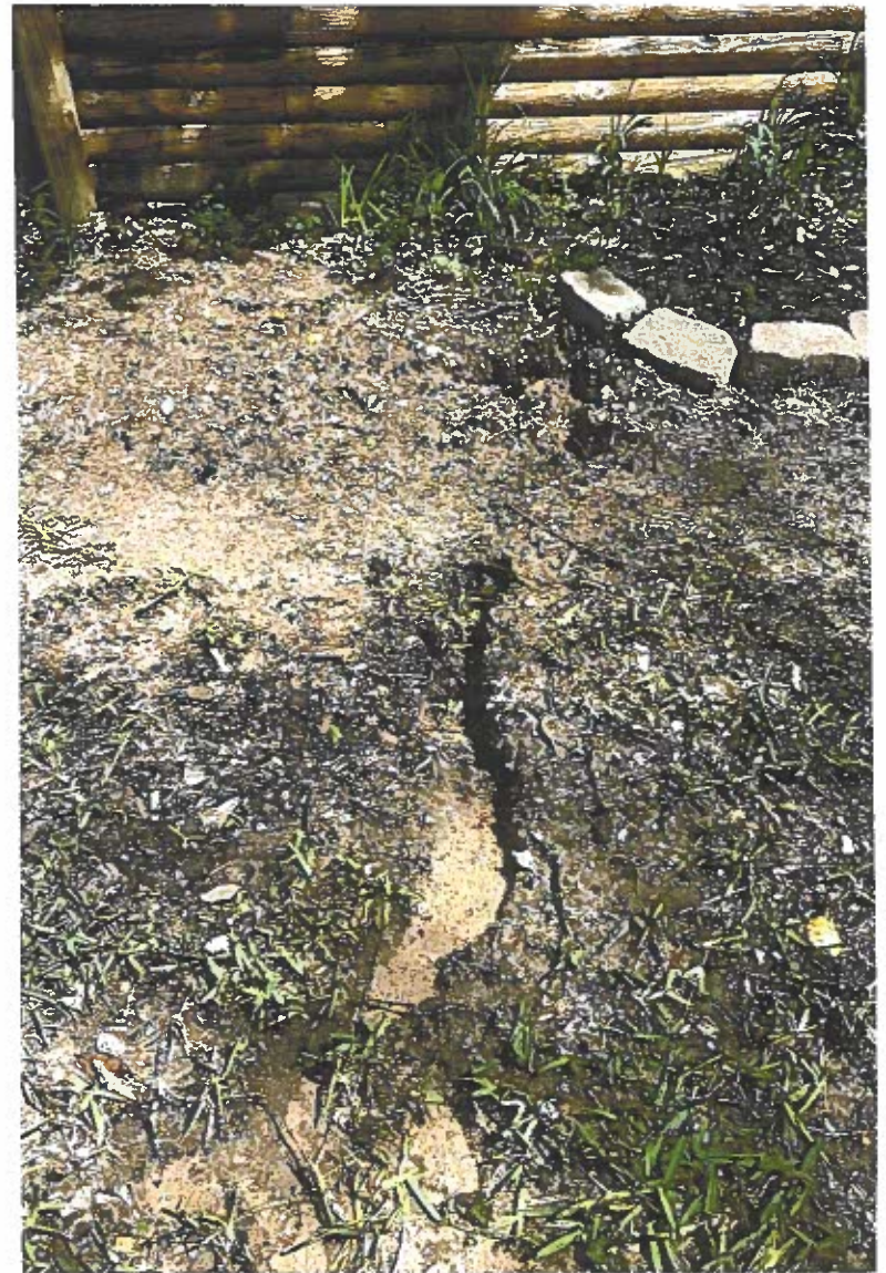
Water comes over and under retaining wall
