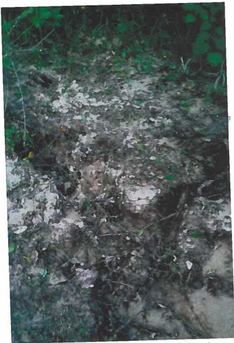
ONE OF MANY WASHOUTS THAT HAS TO BE FILLED AFTER STORMS.
