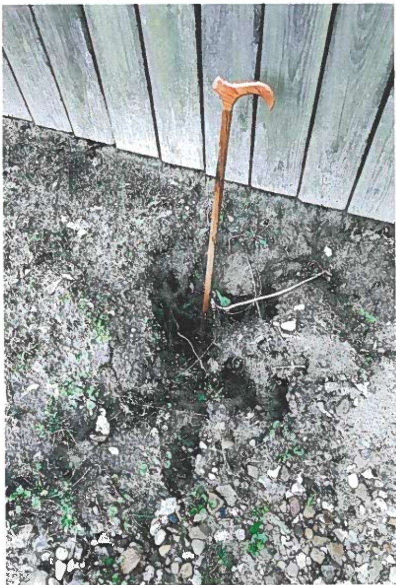
WASHOUTS AND SINKHOLES FORM
