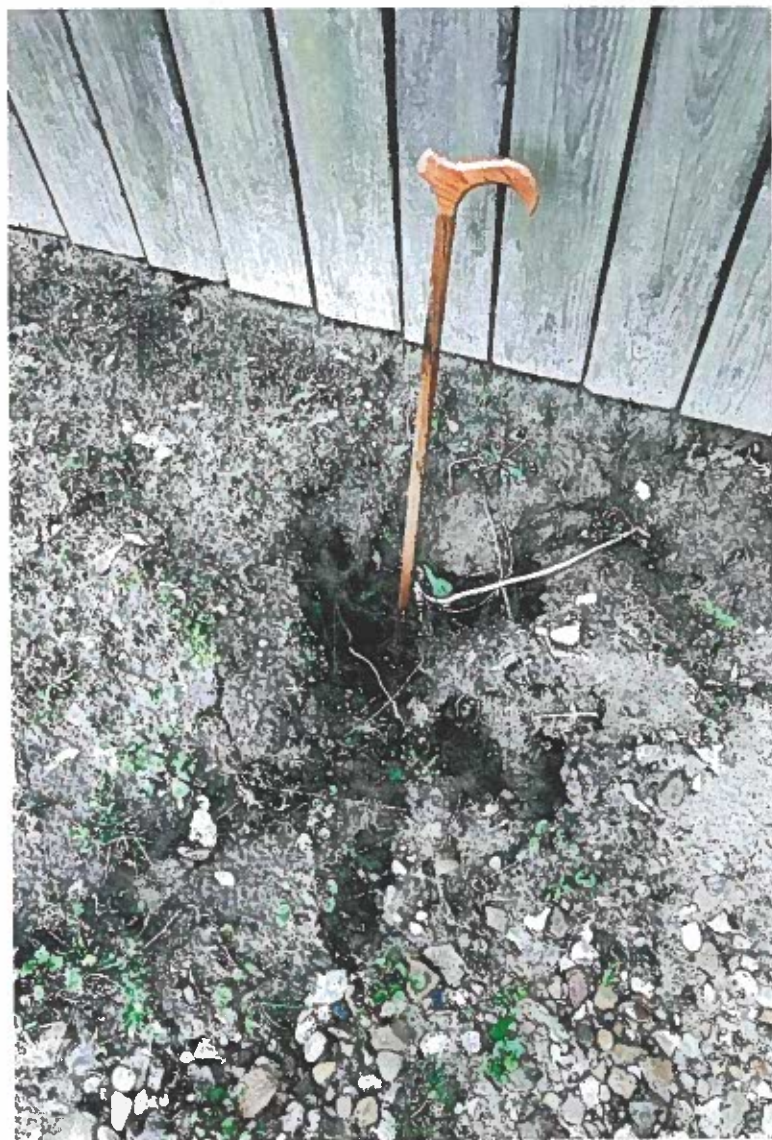
WASHOUTS AND SINKHOLES FORM
