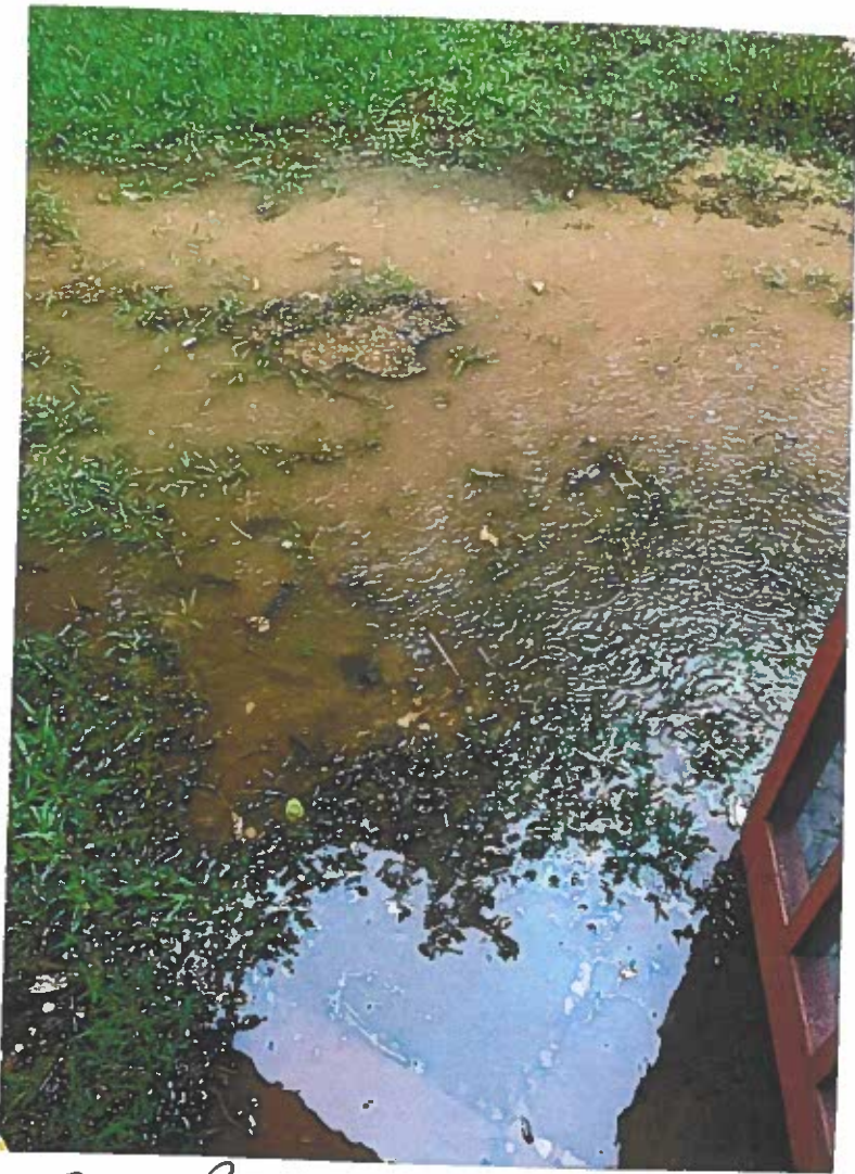
BACK PORCH FLOODING 4-13-2022
