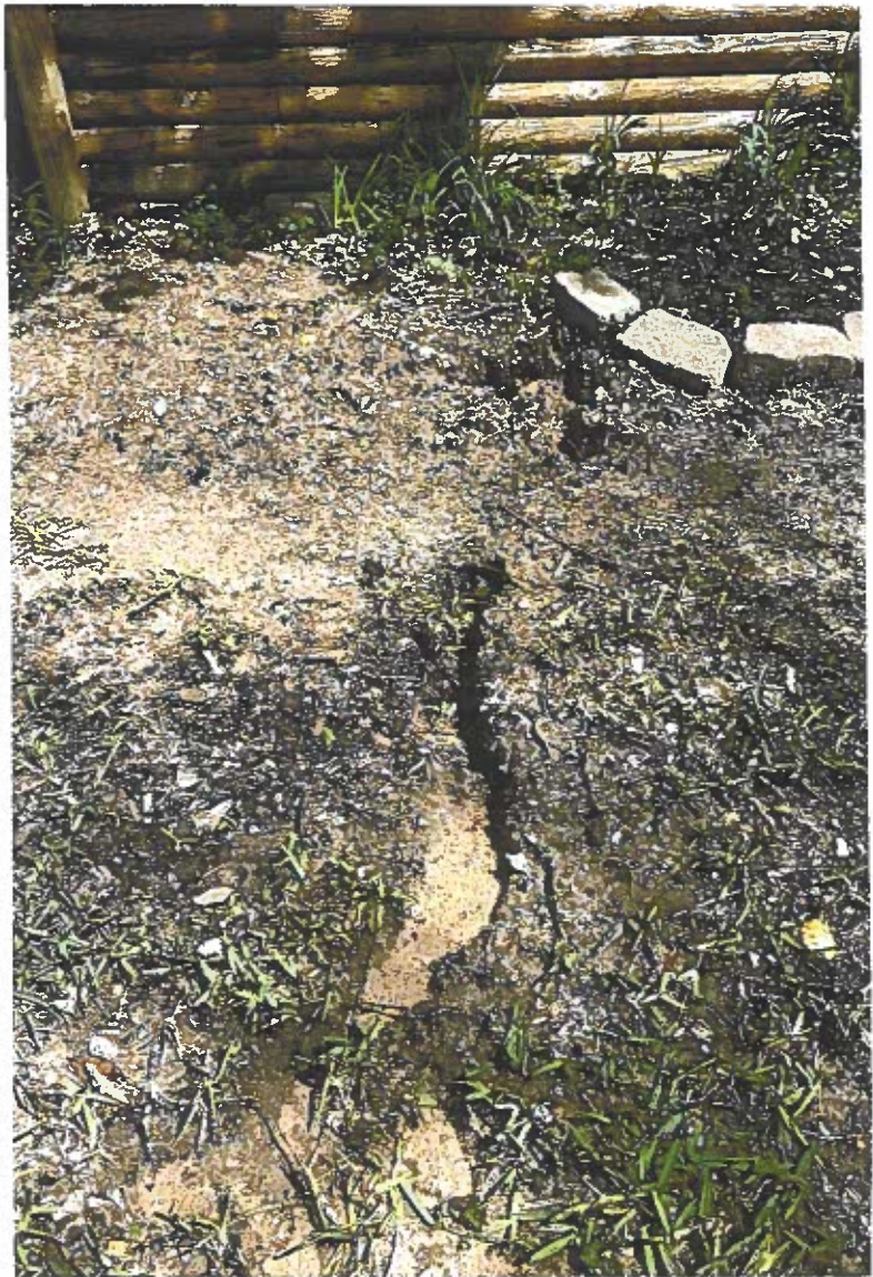
WATER COMES OVER AND UNDER RETAINING WALL
