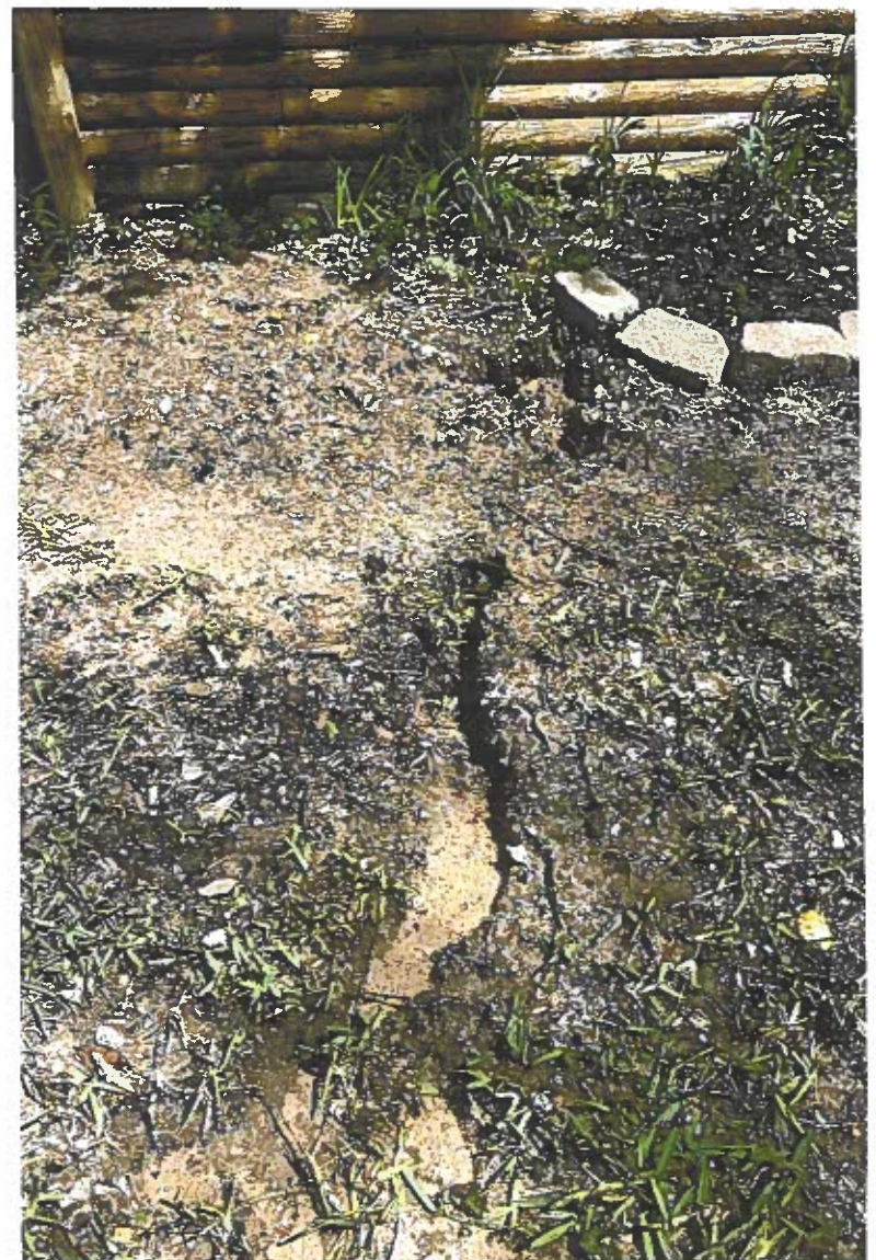
WATER COMES OVER AND UNDER RETAINING WALL
