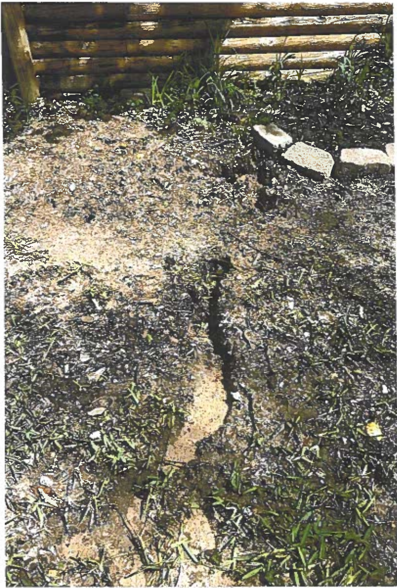
WATER COMES OVER AND UNDER RETAINING WALL
