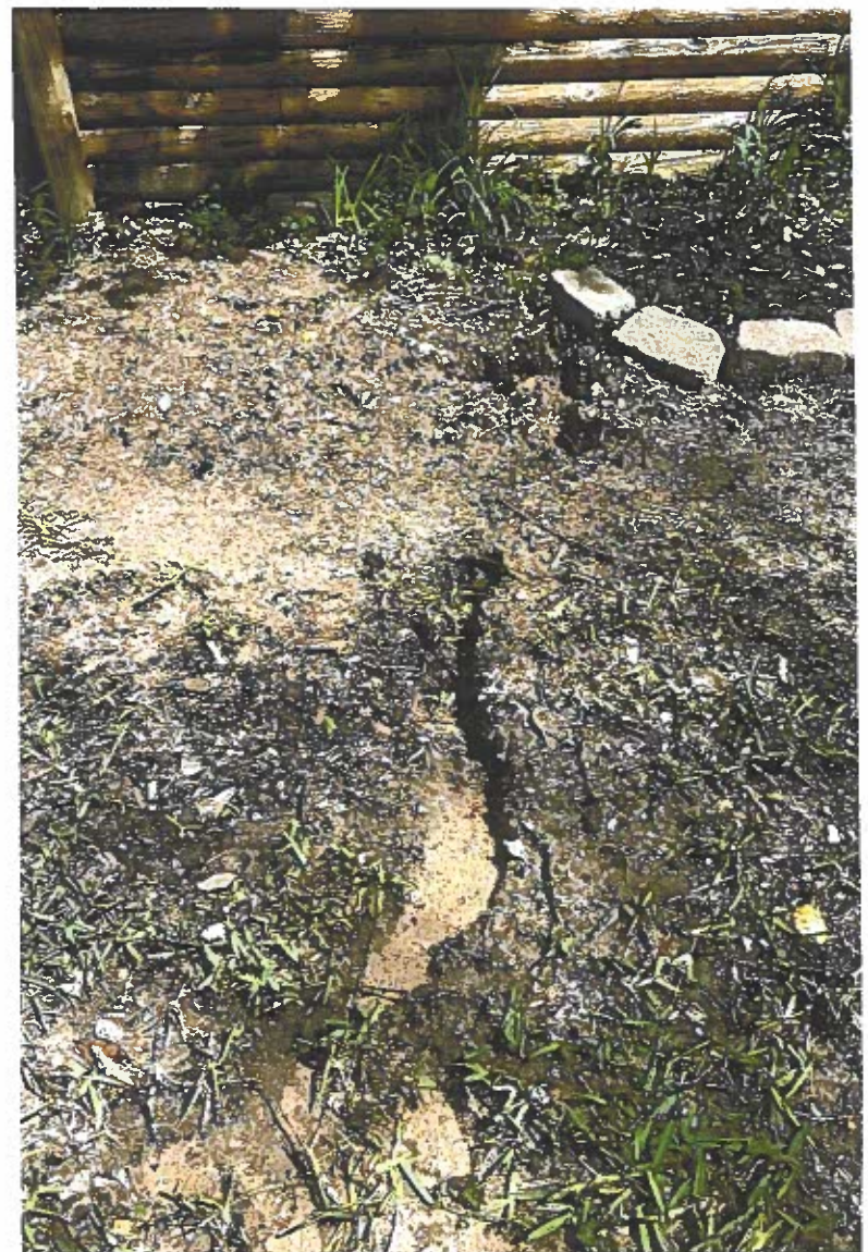
Water comes over and under retaining wall
