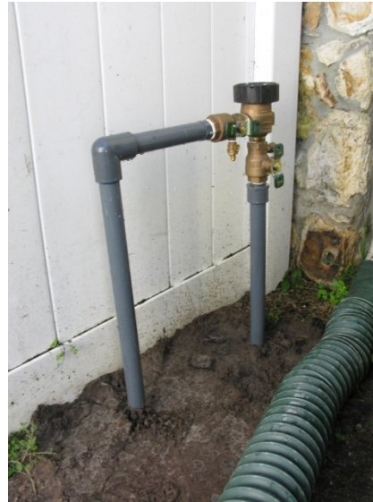
VACUUM BREAKERS & DOUBLE CHECK VALVE BACKFLOW DEVICES
