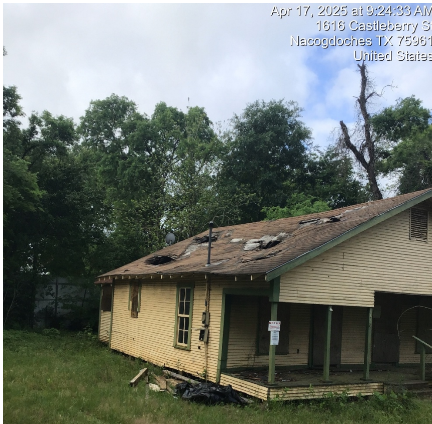
View of structure showing roof damage. Photo taken April 17, 2025.
