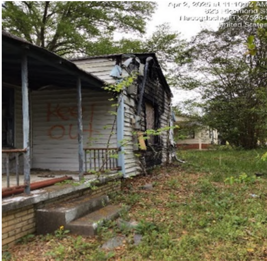
View of structure showing damage. Photo taken April 2, 2025.
