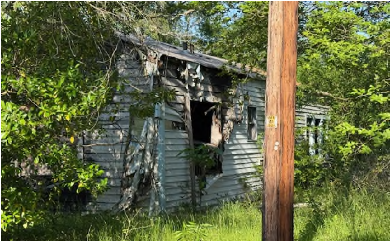
View of structure showing damage. Photo taken April 16, 2025.
