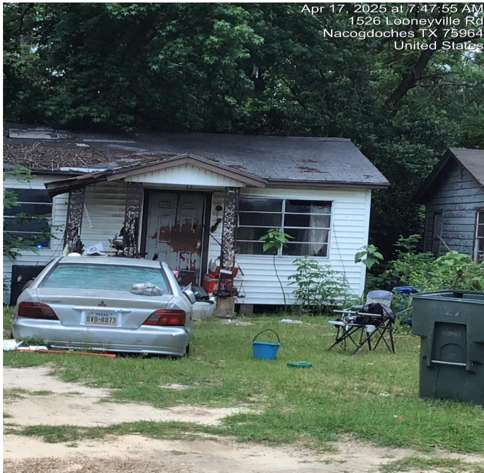
View of structure with plywood over hole roof. Photo taken April 17, 2025.
