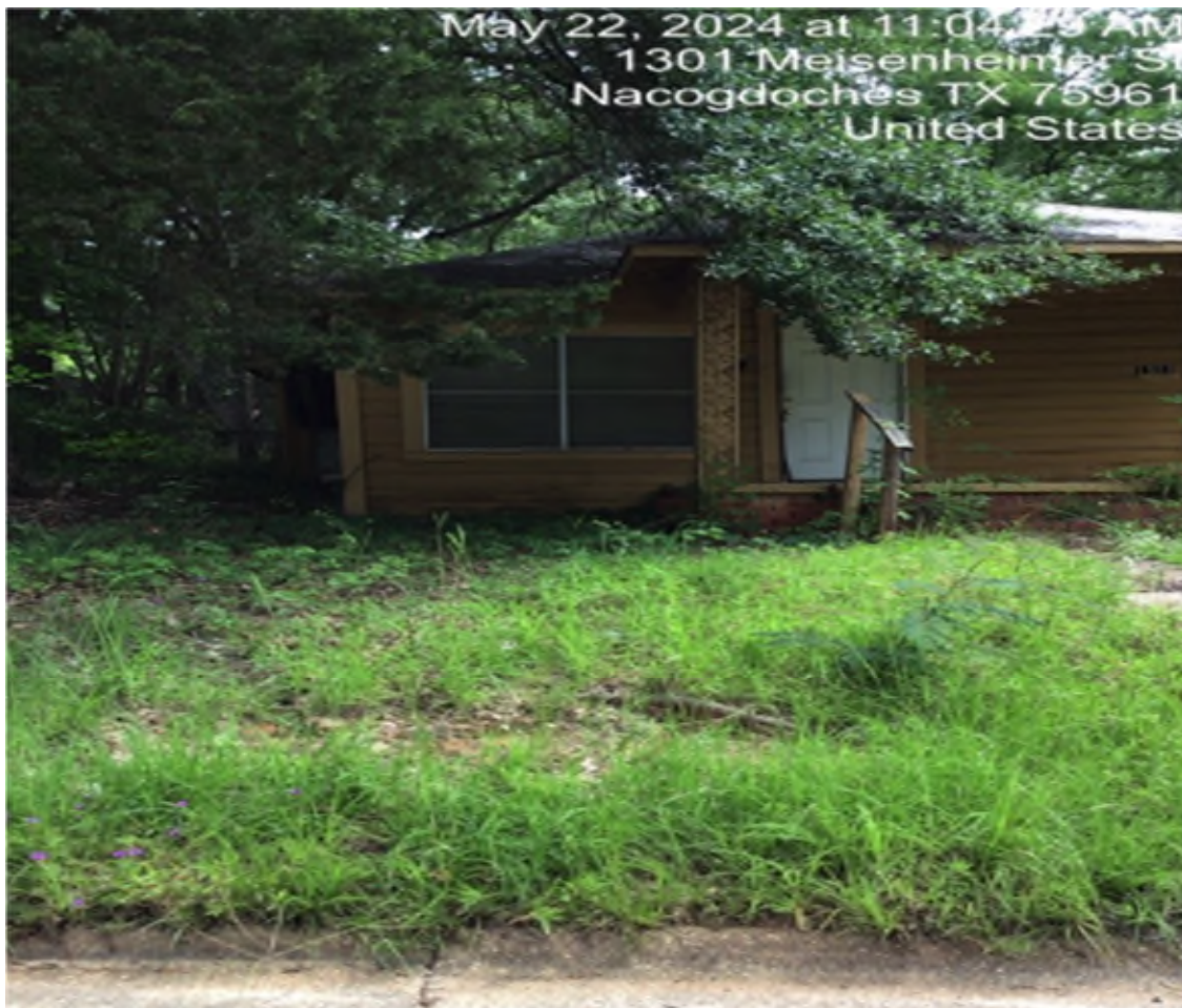
View of structure frontage showing unsecured door. Photo taken May 22, 2024.
