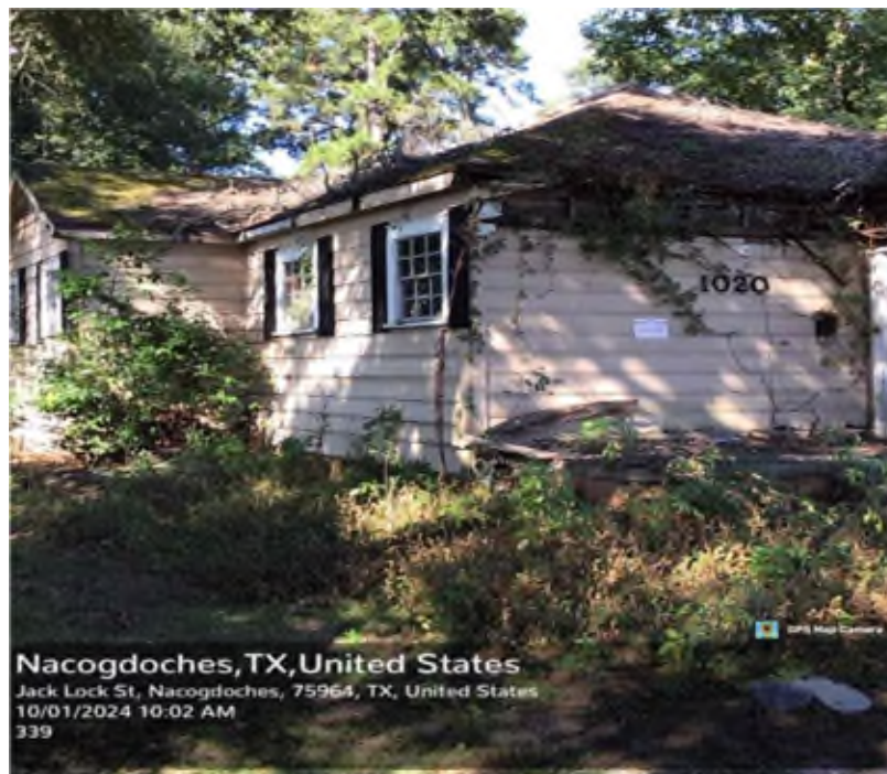
View of structure with limbs and debris on roof. Photo taken October 1, 2024.
