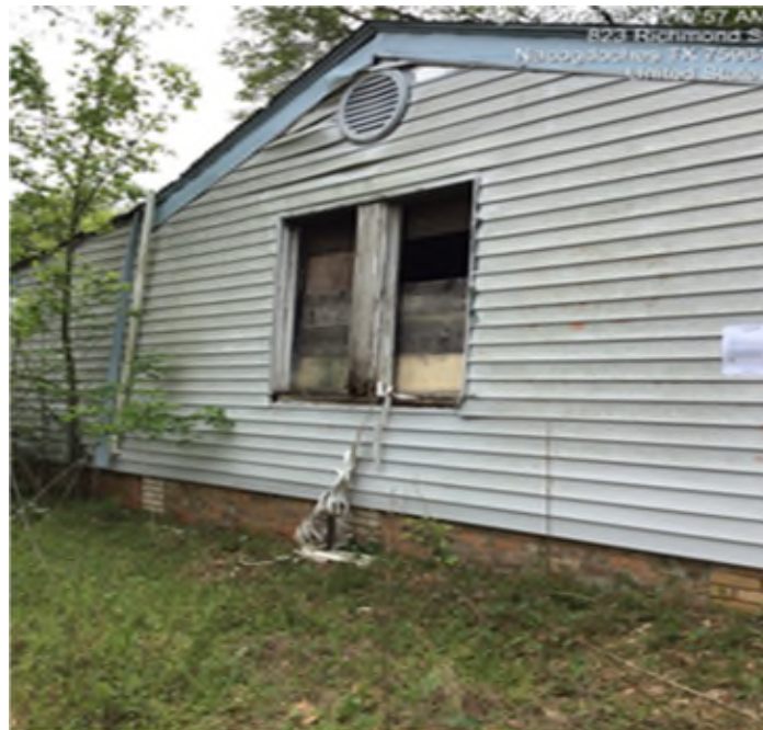
View of structure showing windows broken. Photo taken April 2, 2025.
