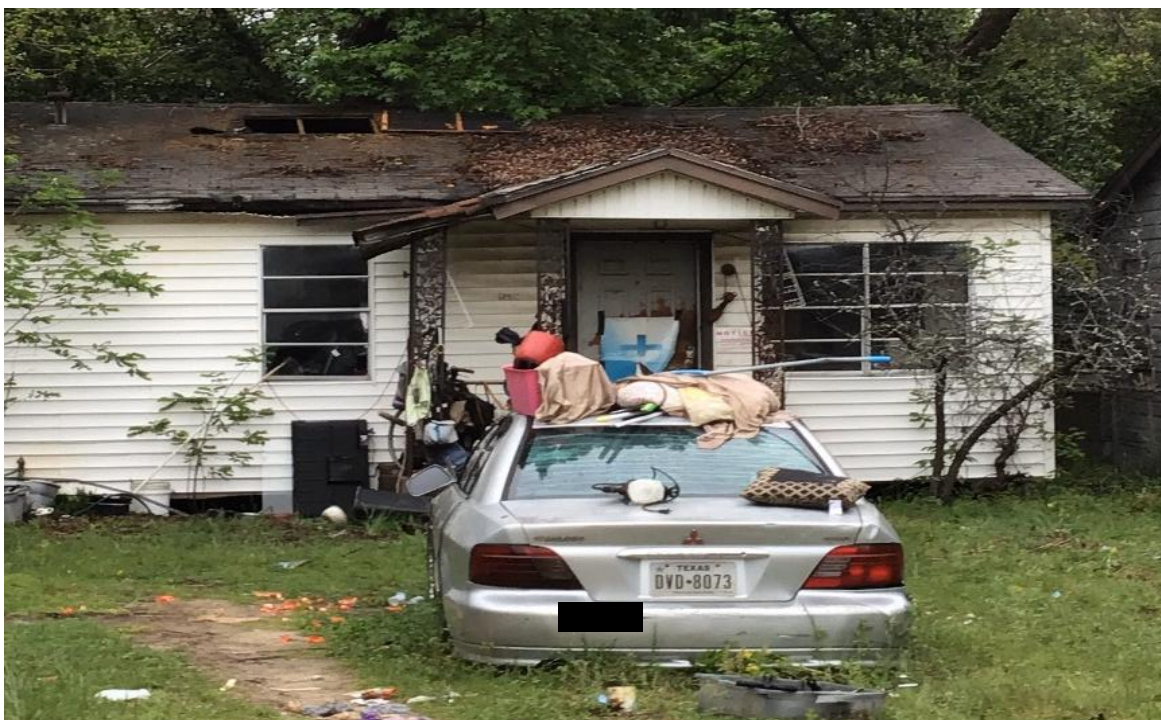
View of structure with hole in roof. Photo taken March 21, 2024.
