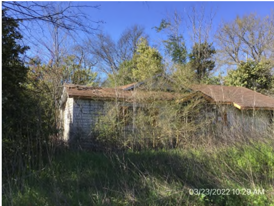
View of structure frontage with tree limbs on roof. Photo taken March 23, 2022.
